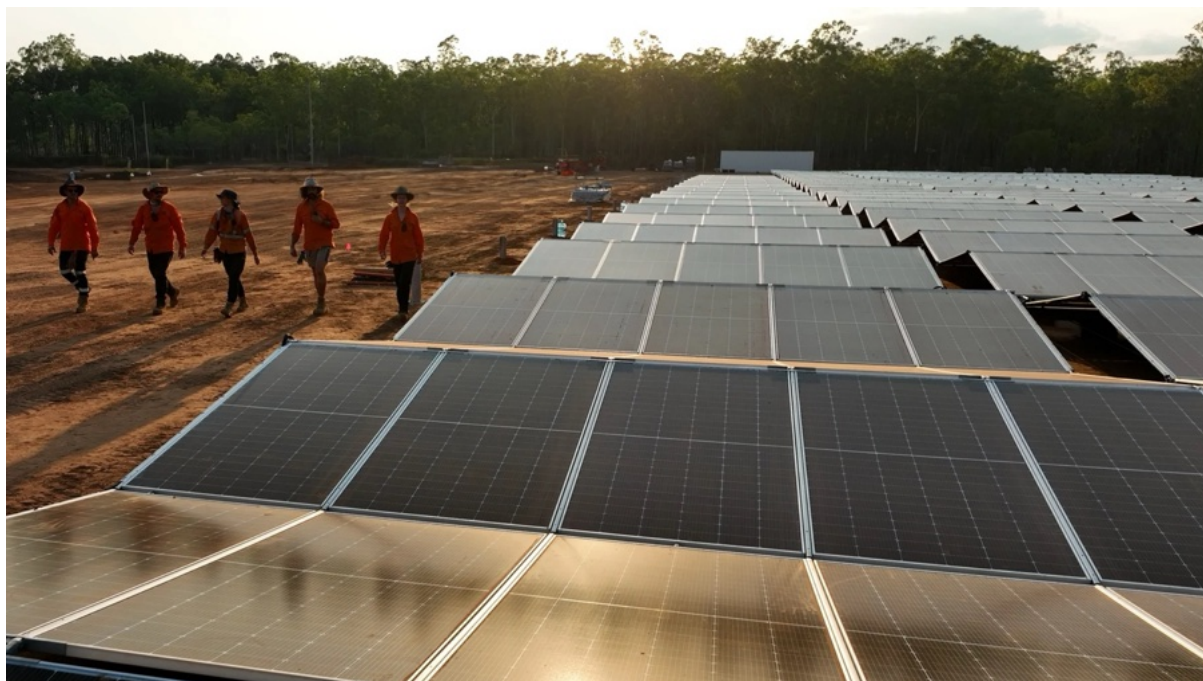
Figure 1 5B Maverick solar array system
