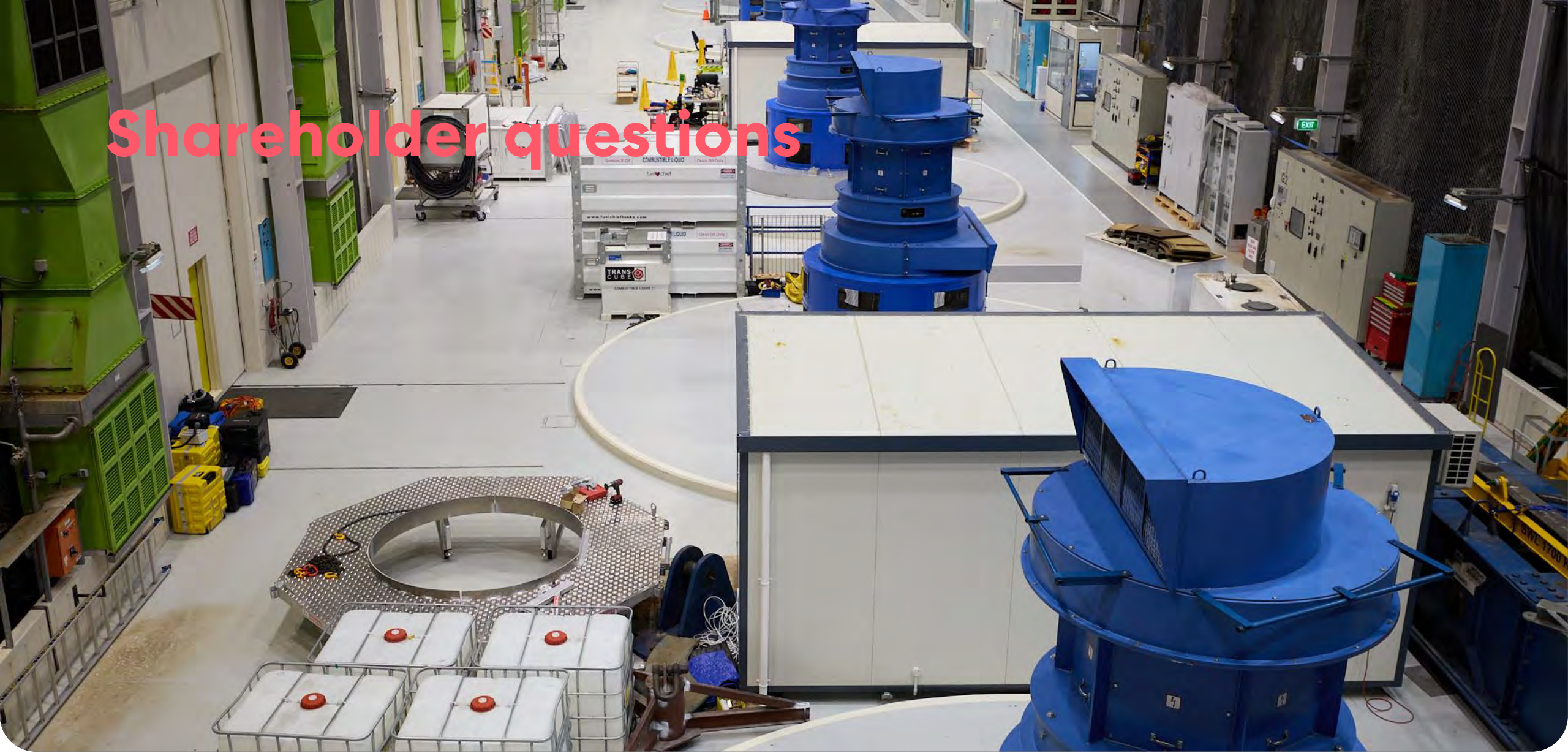
Manapouri Power Station in Fiordland.
