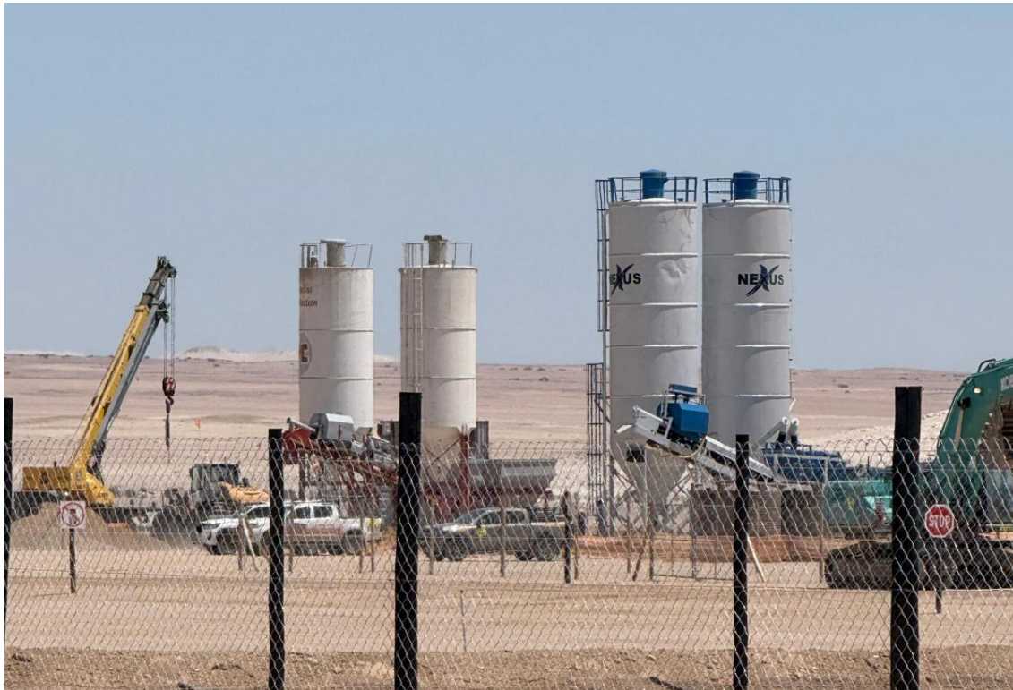
Figure 7: Concrete Batching Plant
