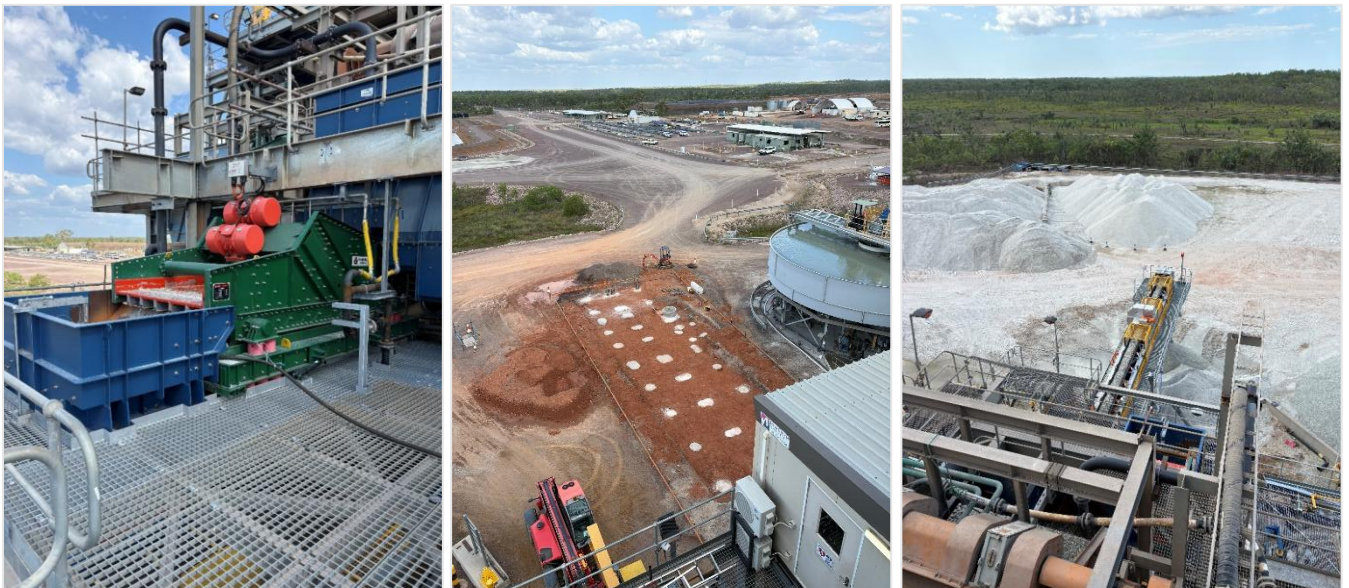
Figure 4 DMS plant brownfields modifications (Left to right) 1. Upgraded rolls crusher screen. 2. Reflux classifier pad. 3. New middlings conveyor
