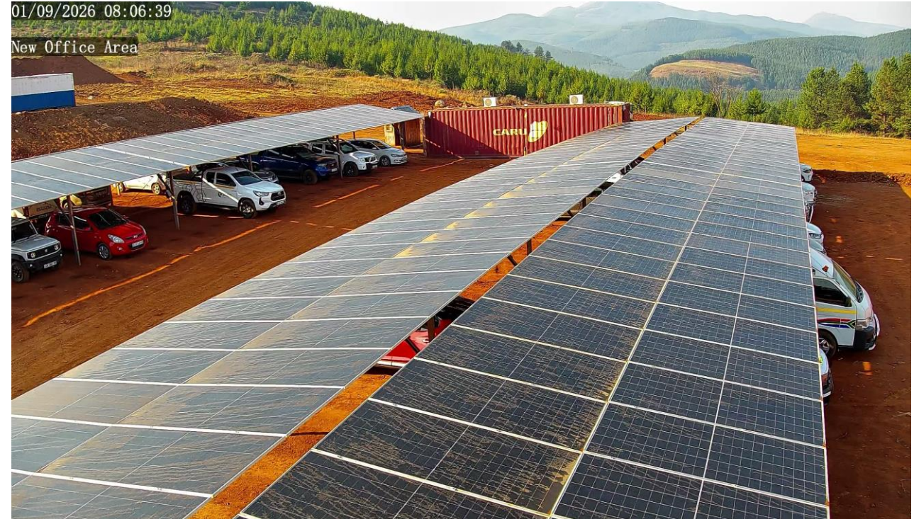
Solar Car Park and Battery System
