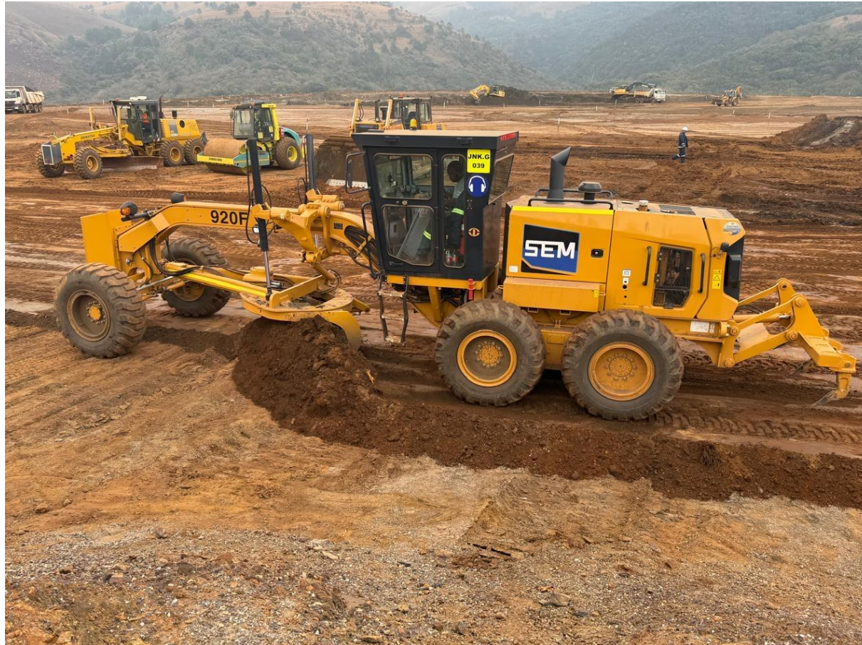
Tailing Facility System
