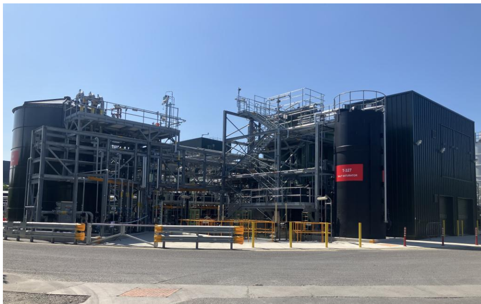
PHOSPHIX® phosphate removal plant, delivered in partnership with Enva in Ireland.
