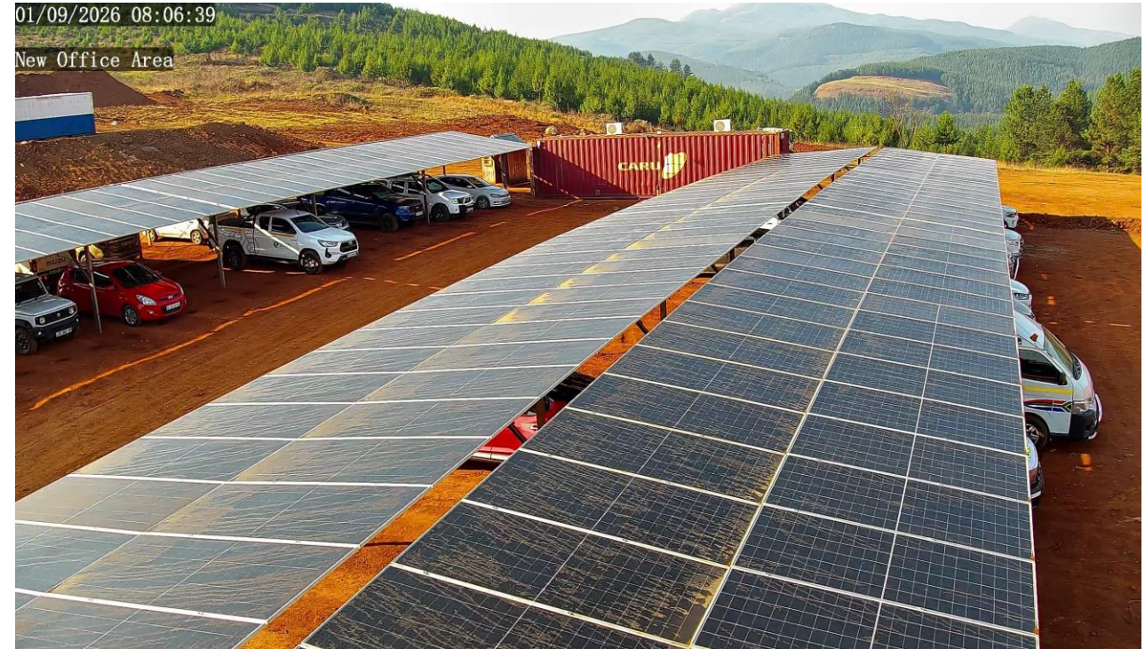
Solar Car Park and Battery System
