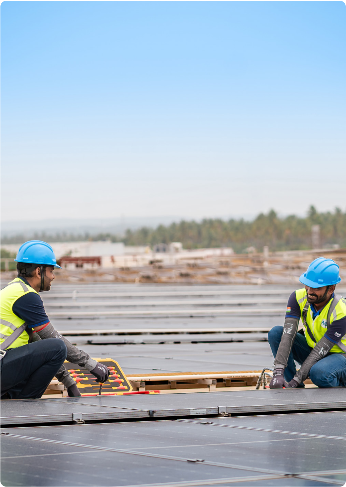
↑ Image caption: Employees at Ansell's India manufacturing site carry out maintenance activities on the site's solar panel system.
