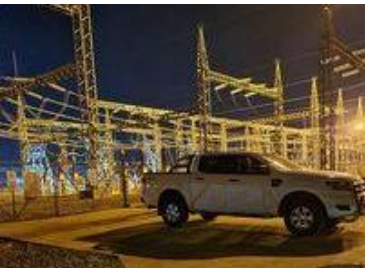
Eskom Power Substation 12km away
