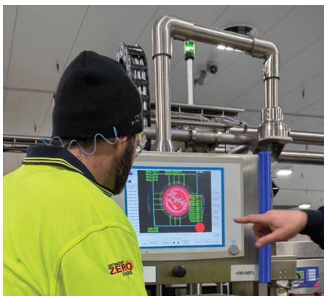
Example of assistive technology installed in our Barossa Packaging Centre.
