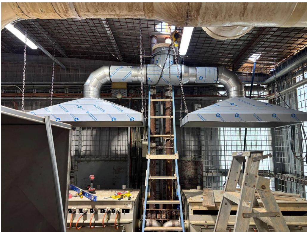
Figure 3: Fume hoods installed in gold room
