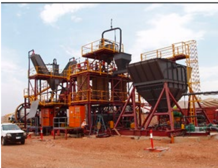
Photo 2: Modular Gravity Plant Installed and operational (as previously operated)
