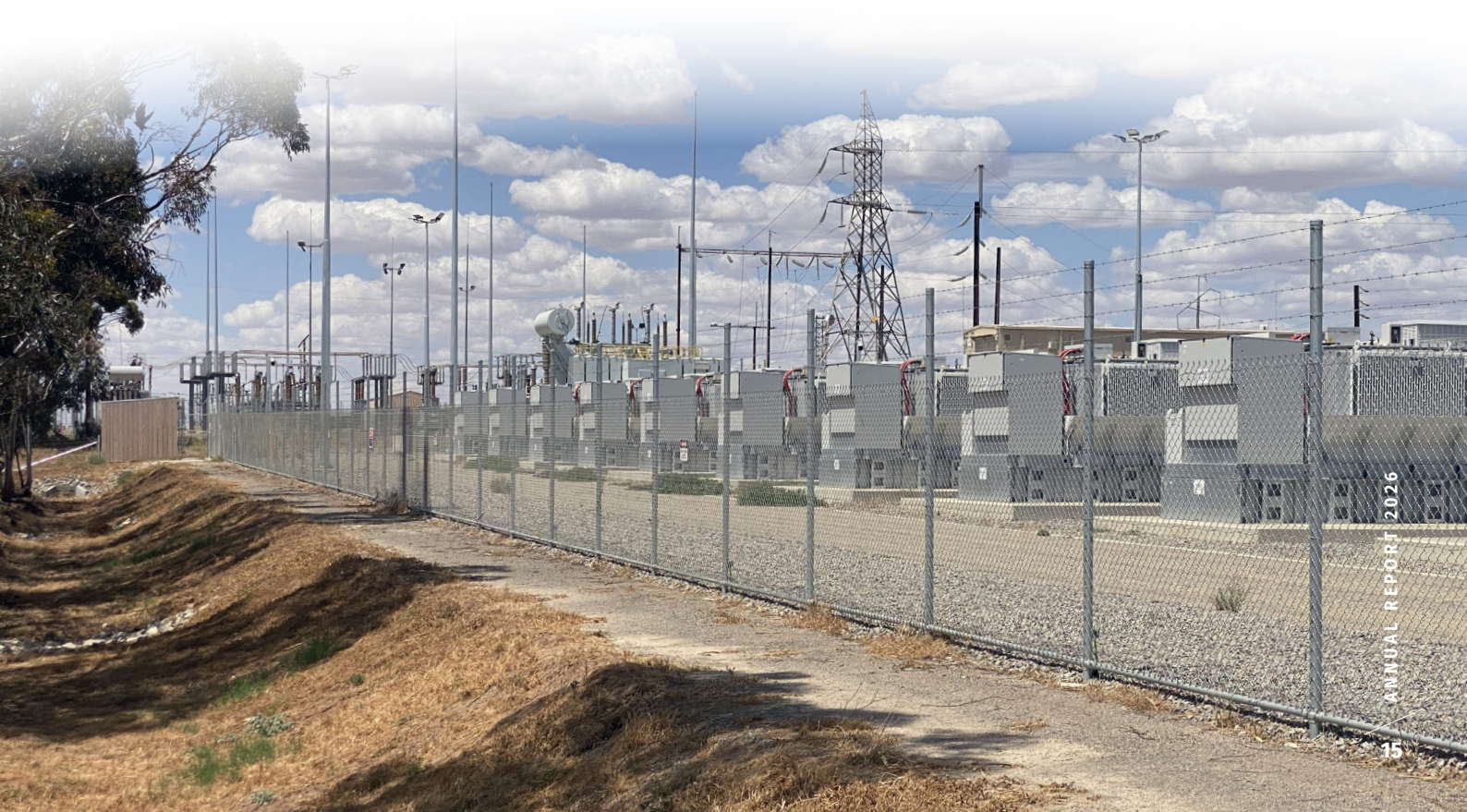
Battery Energy Storage System, Monarto Energy Project, South Australia.
