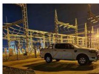
Eskom Substation 12km away
