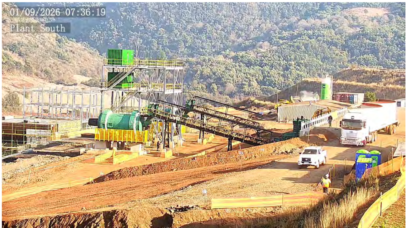
Figure 34: Twin ball mills installed with conveyor feed system and supporting process infrastructure
