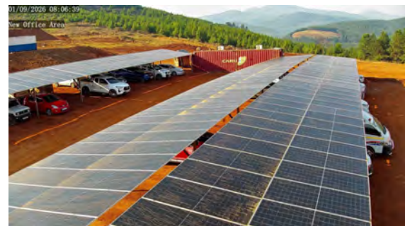
Figure 21: Solar power car park and battery system
