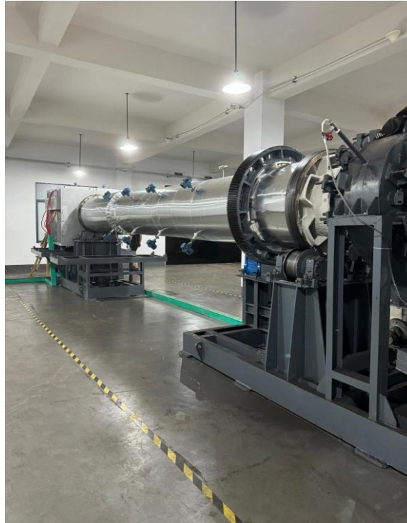
The Company's High-Efficiency Energy-Saving Roasting and Drying Kiln at Firebird's pilot plant, Hunan, China
