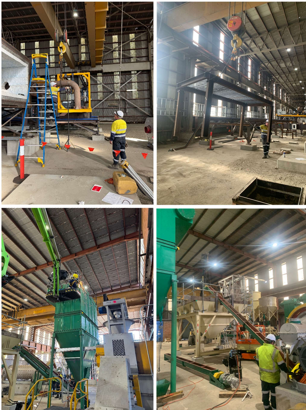
Figure: SMP activities in Reduction Furnace (top) and Briquetting (bottom) areas.
