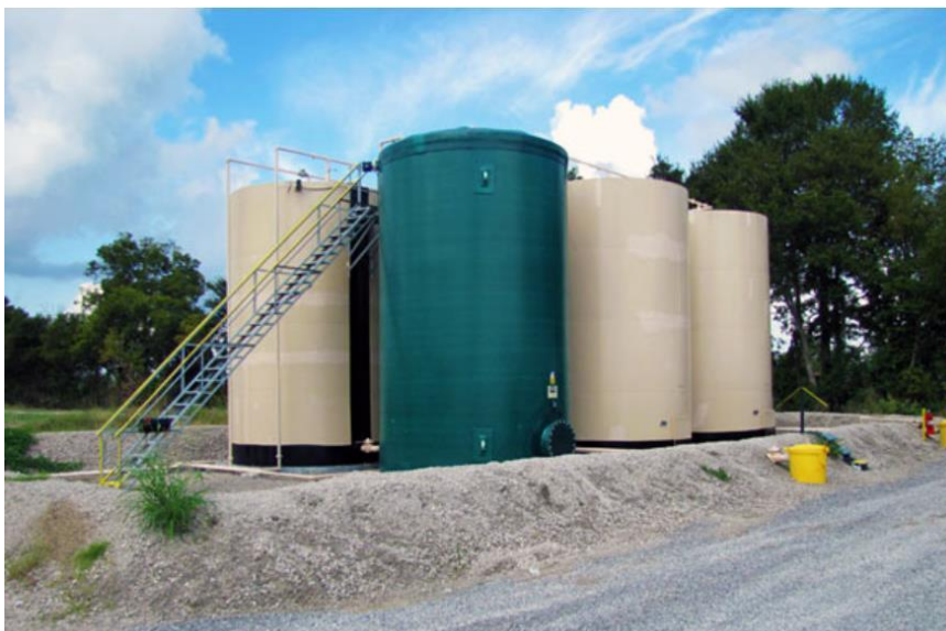
Figure 1: Hensarling #1 well oil storage tanks, Desiree Field, Louisiana.
