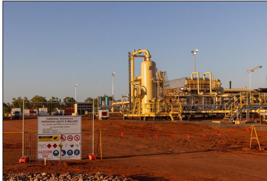
Sturt Plateau Compression Facility (September 2026)
