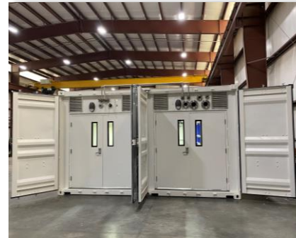
Modular emulsion plant
