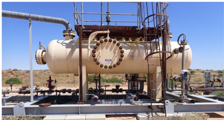
Gas/liquids separator in place at Vanessa facility
