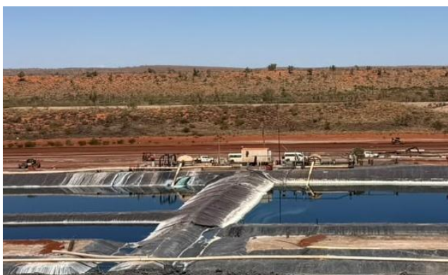
ILS2 and PLS2 pump station commissioning
