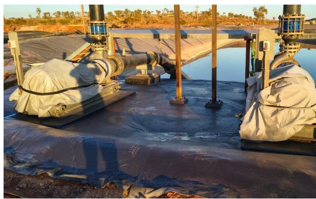
Containment infrastructure around pumps
