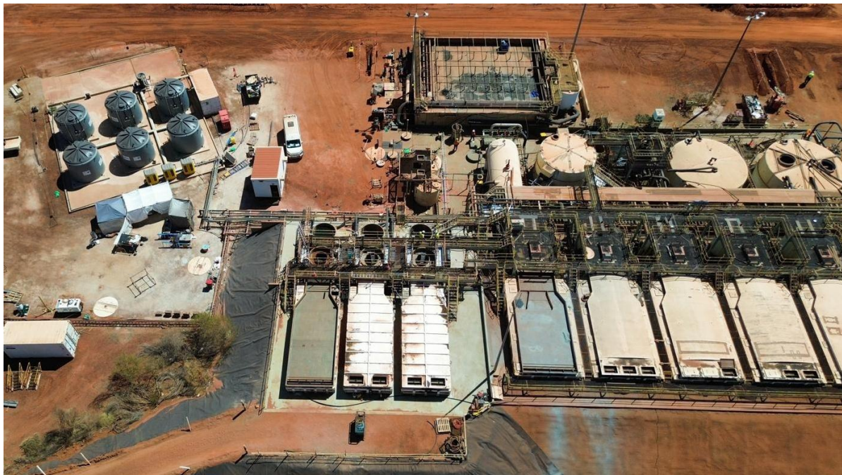
Solvent Extraction Plant Area (SX)
