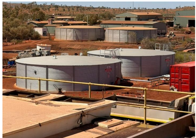
Firewater system installed
