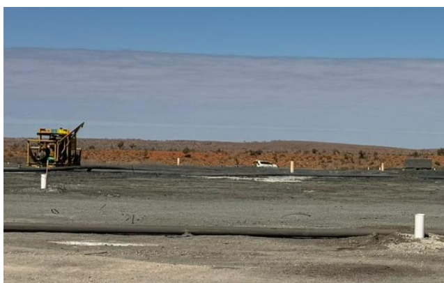
High pressure pump for injection leaching
