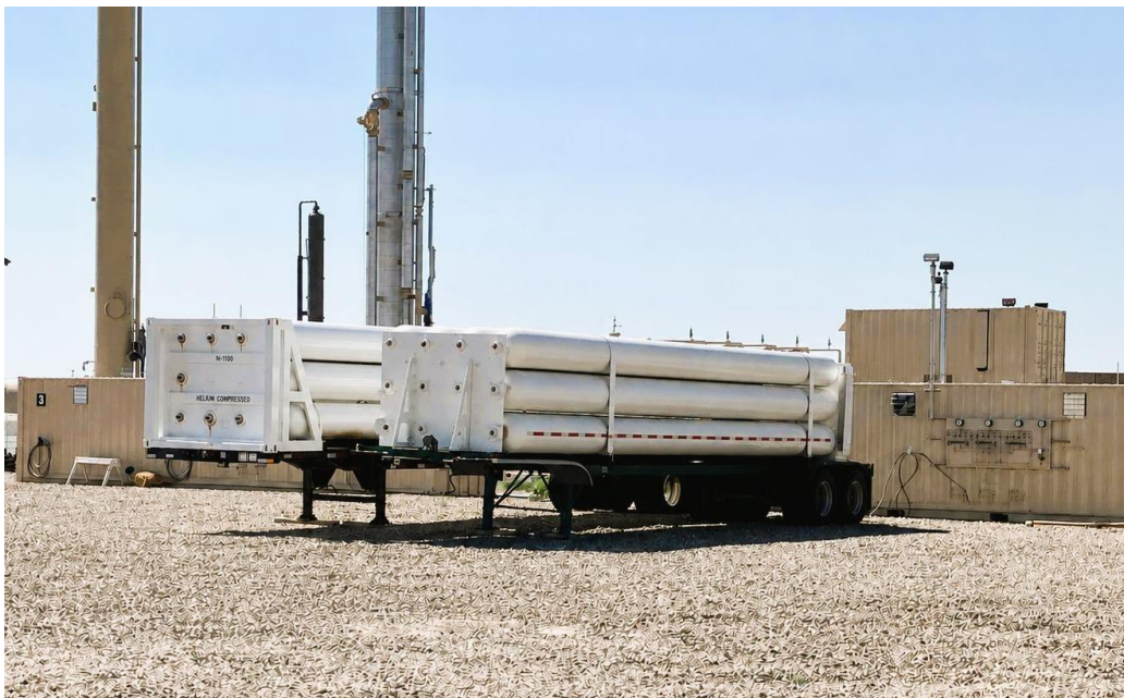
Figure 2: Tube trailers at the Pinon Canyon Plant
