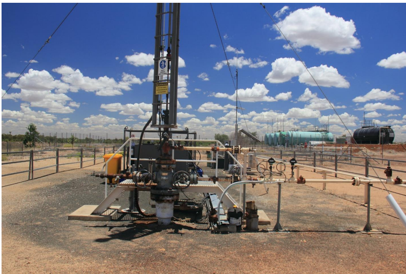
Figure 2: Wellhead and storage infrastructure at Emu Apple-1, PL 264
