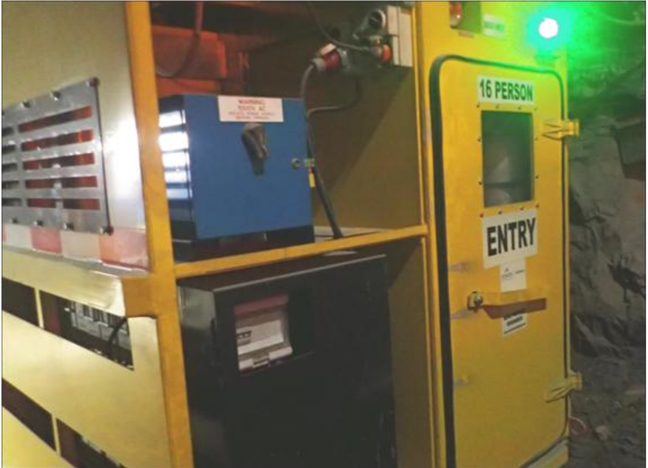
Figure 16-9: Typical underground refuge chamber
