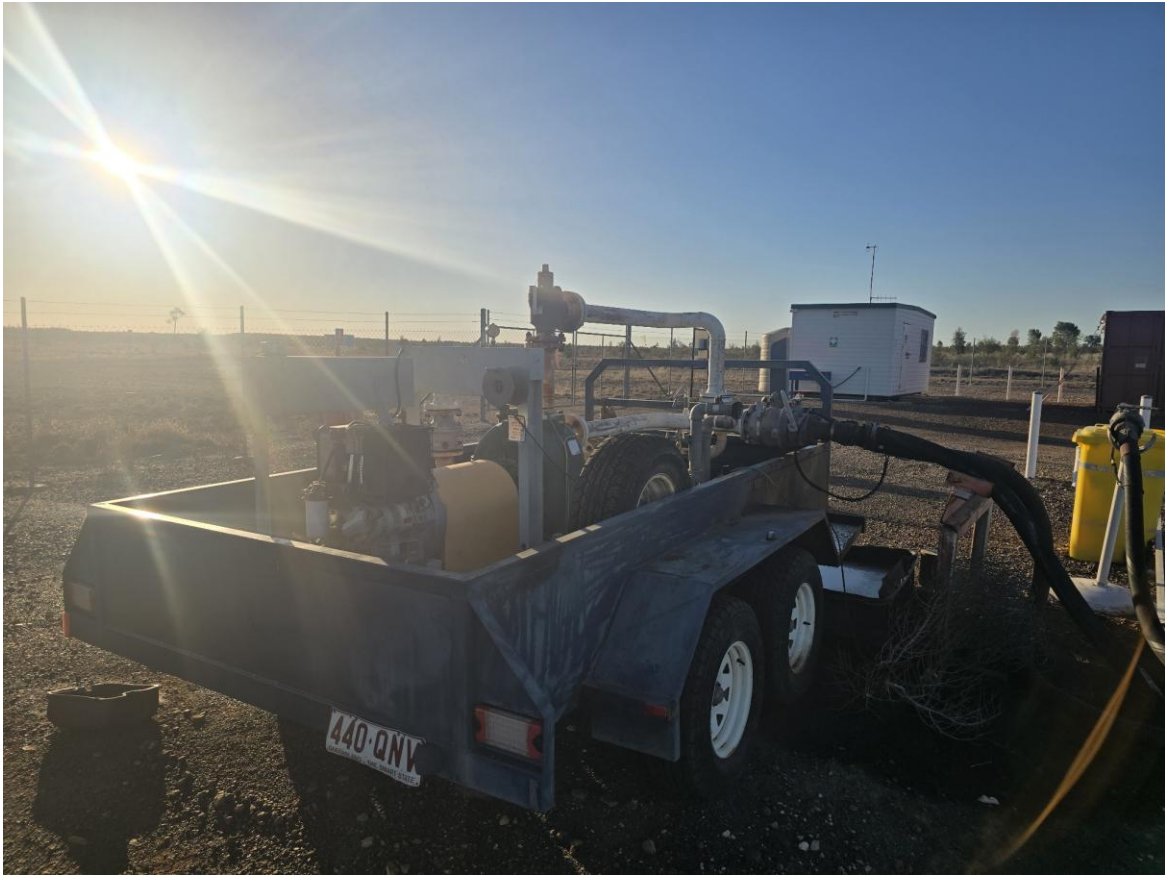
Figure 3 Load out pump on trailer at Emu Apple in readiness to be mobilised to the Riverslea Field
