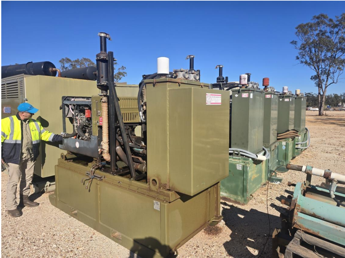
Figure 1 Emu Apple-1 operations have provided scope to utilise the existing evaporation ponds to bring on other wells. Exploration and Development Manager Len Diekman inspecting the additional hydraulic units planned to be deployed into Emu Apple and Riverslea fields.
