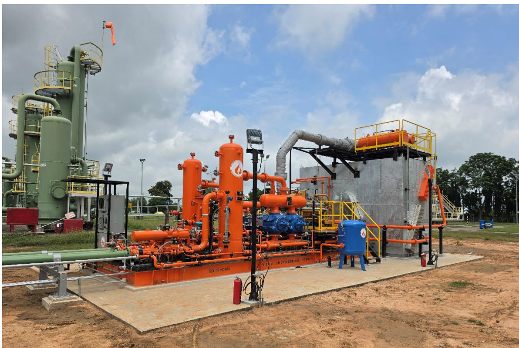
Figure 1: Nam Phong Booster Gas Compressor
