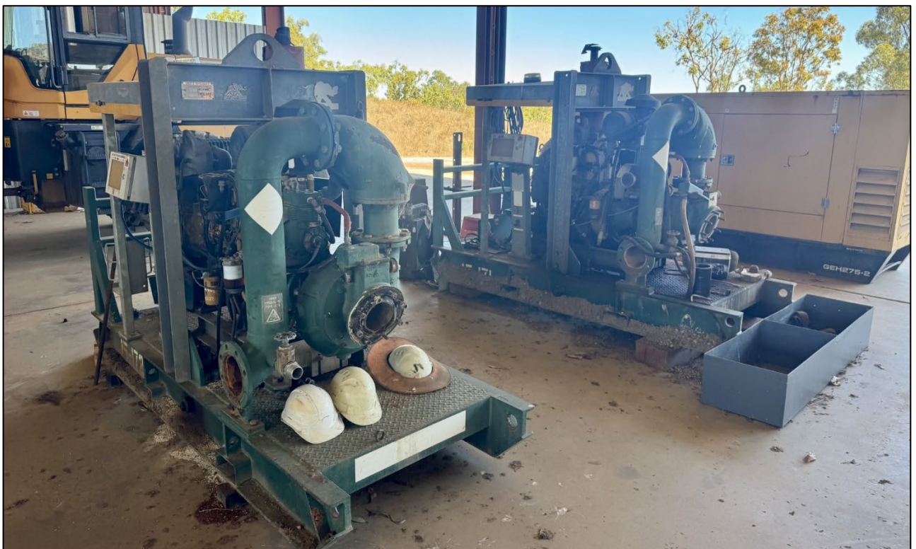
Figure 5: Water pumps in workshop ahead of reconditioning.
