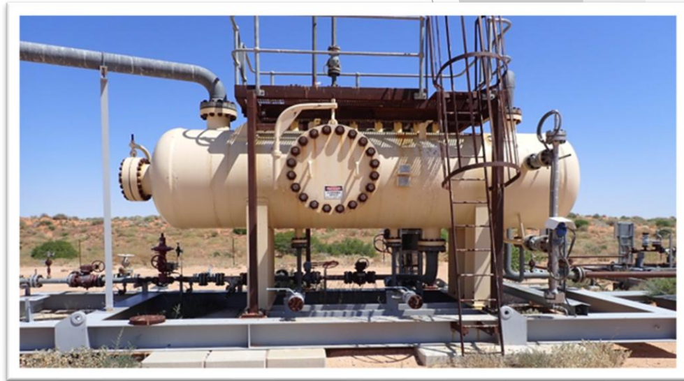
Gas/liquids separator in place at Vanessa facility
