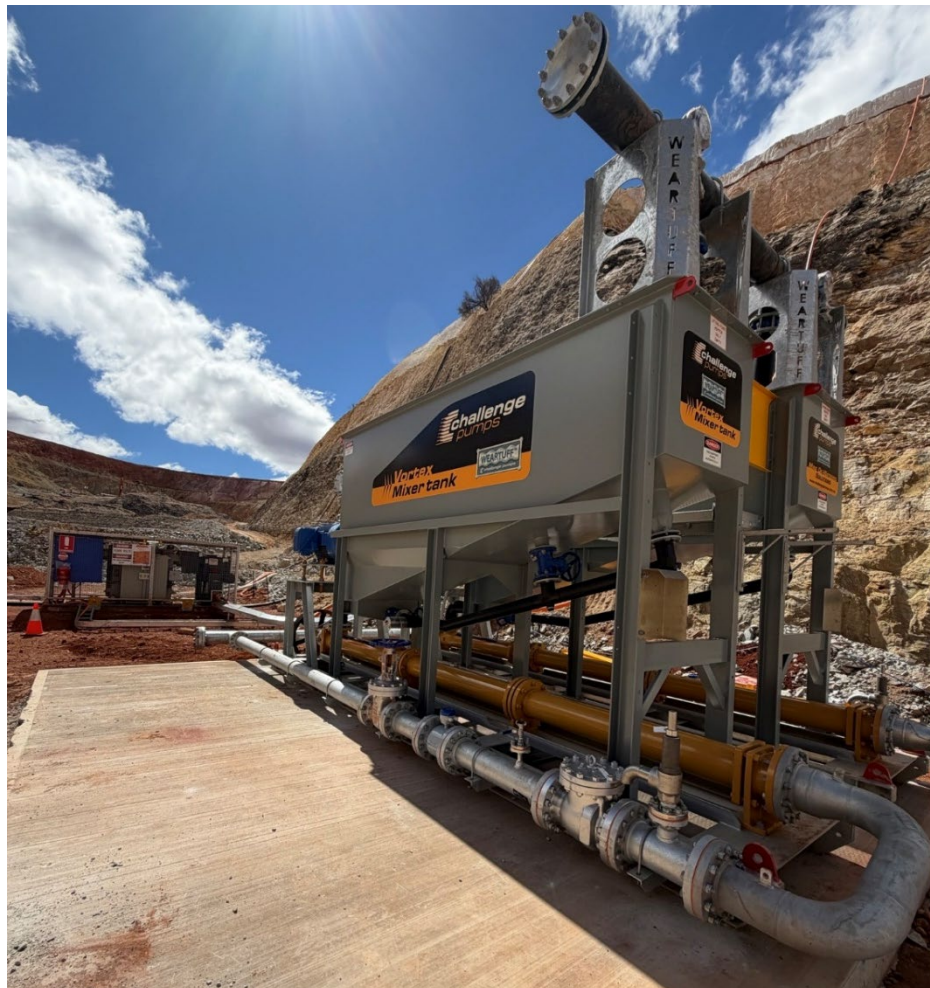
Figure 9 – Youanmi Main in-pit pump station
