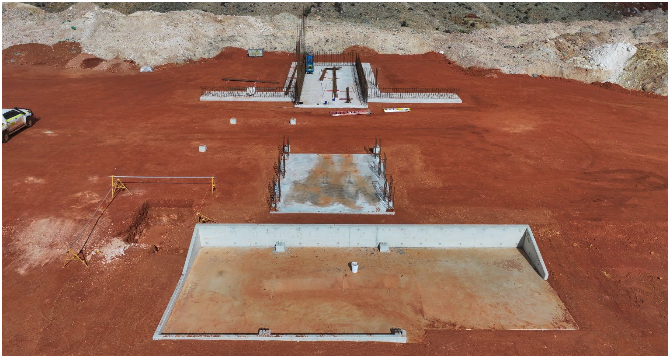
Figure 2 – Crushing circuit – primary crusher pad in background, secondary/tertiary crushers in middle, transfer station at front
