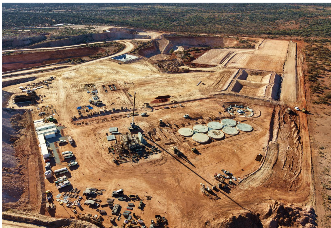
Figure 4: Laverton Processing Plant site (July 2026)
