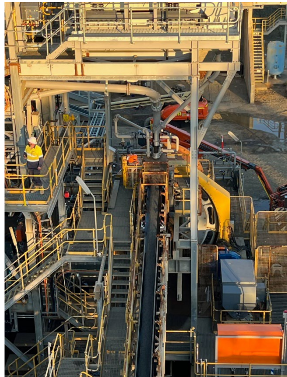
Figure 2 Overhead view of ore belt feeding ball mill
