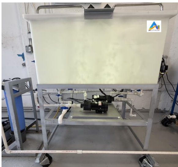
Figure 1: View of the 5 –10gpm Fe removal unit showing sparging in the center of the image.
