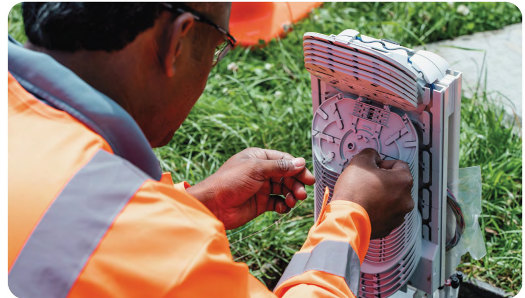
Technician preparing network connections inside a fibre distribution point
