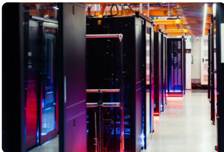
Datacentre220 – our first Express Connect installation
