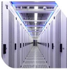
DC Cabinet Security
