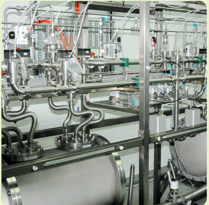
Q-Si Production Plant
