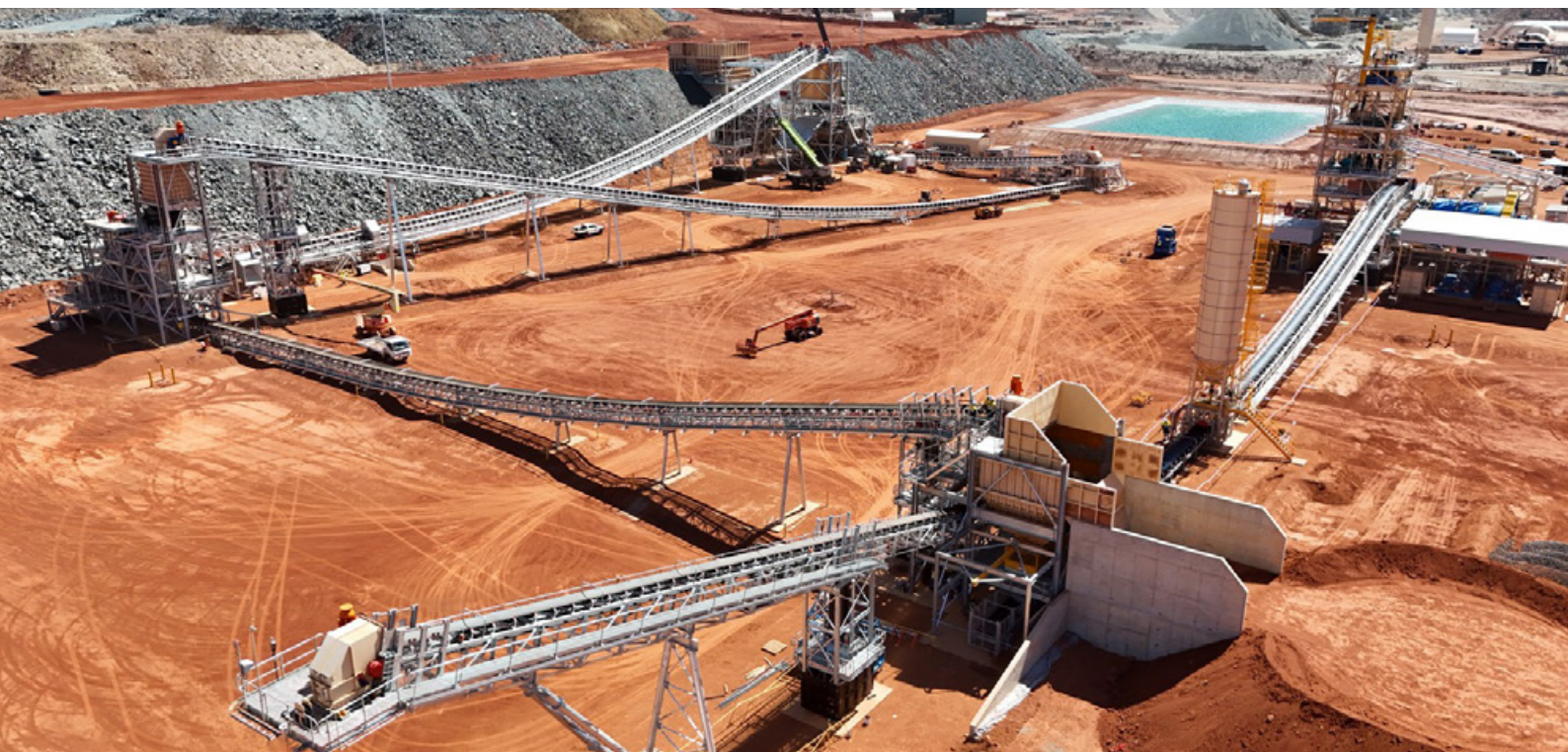
Karlawinda Expansion Project – Surge bin, crushing circuit and ROM2
