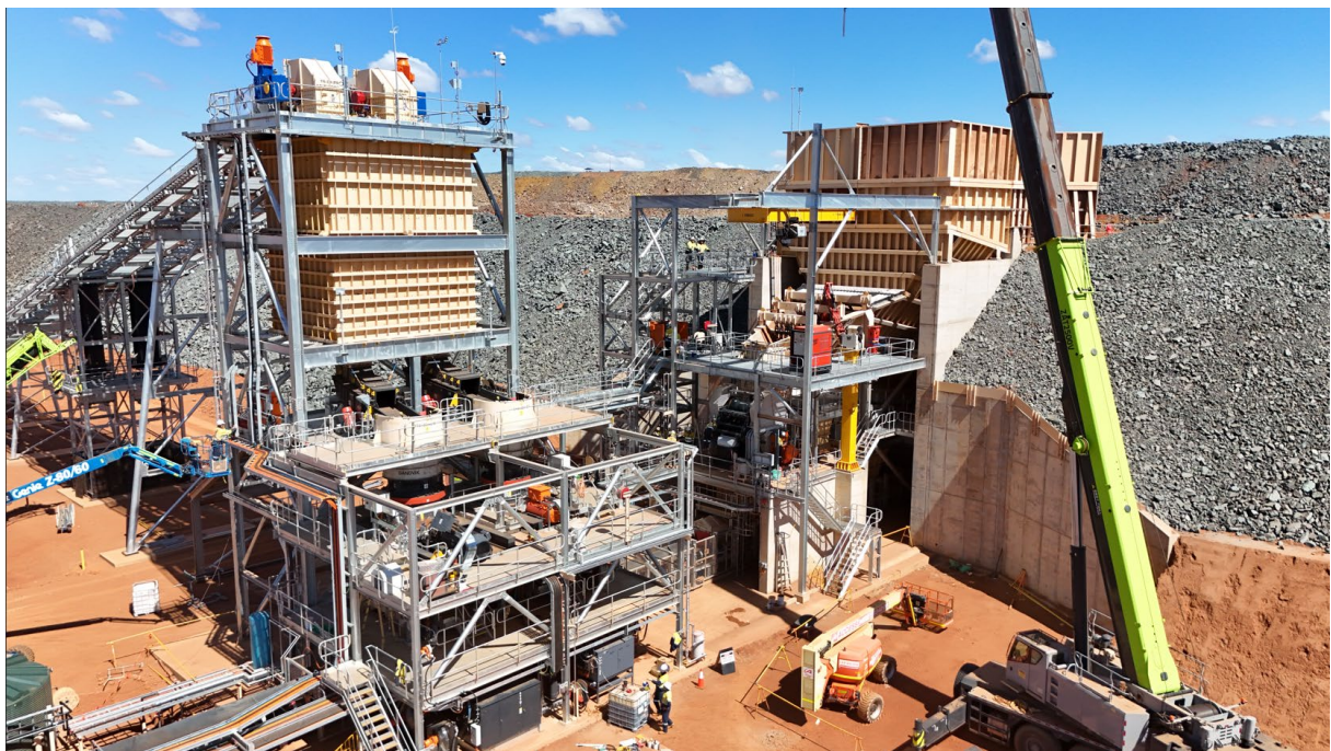
Karlawinda Expansion Project – Primary / Secondary / Tertiary Crushers.
