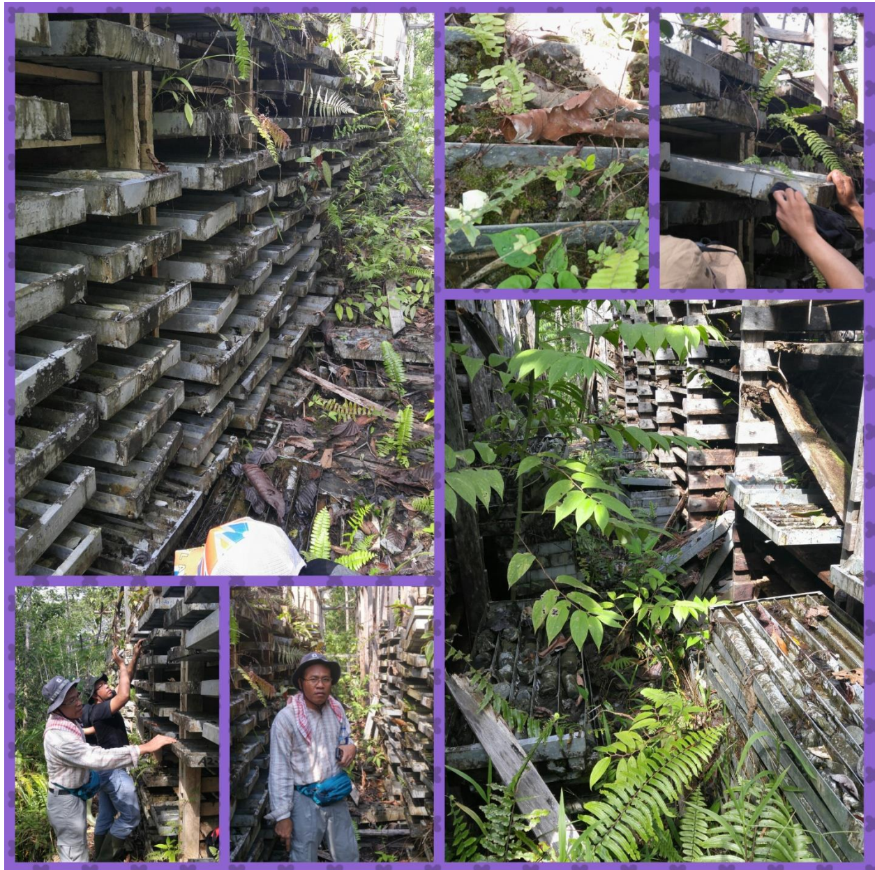
Photo 2. Condition of Tekai Coreshed on 2 November 2016
