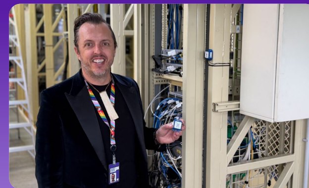
Spark's Autonomous Network Lead, Ulrich Ferik demonstrates a Packet Power sensor which enables real-time power monitoring at the Remuera Exchange.
