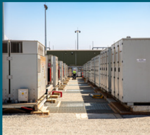
Image: Port Hedland BESS, WA
