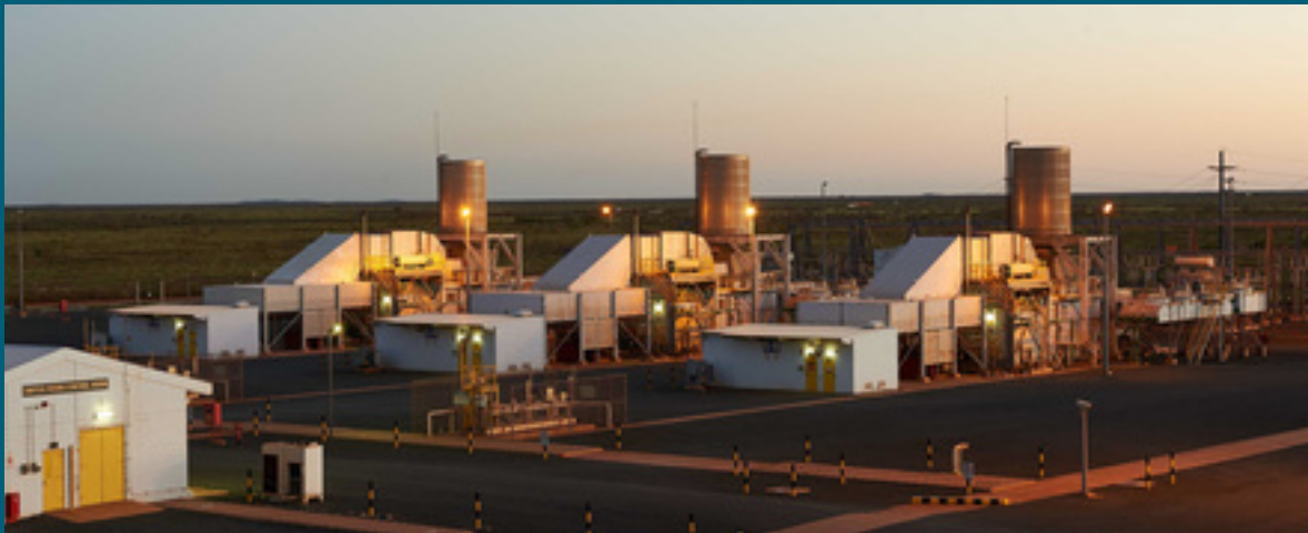
Image: Port Hedland Power Station, WA
