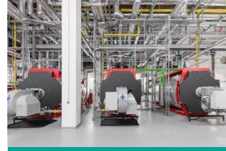
Industrial Package Boiler
