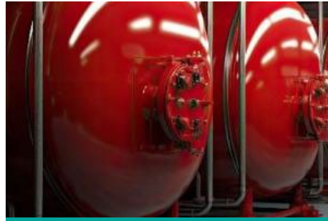
Thermal Oil Heaters
