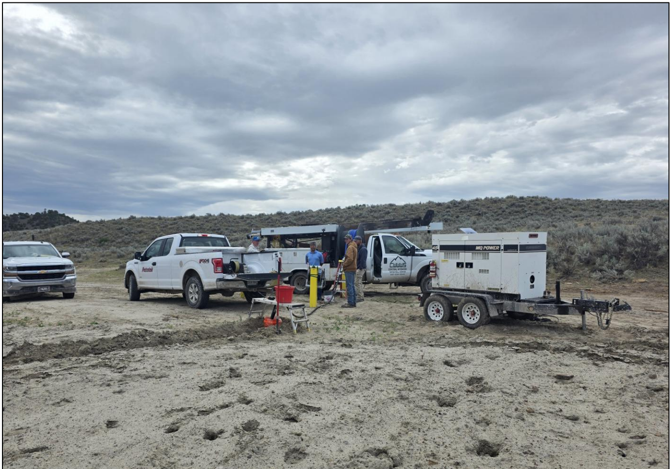
FIGURE 2: LO HERMA MINE UNIT 1 PUMP TEST IN PROGRESS
