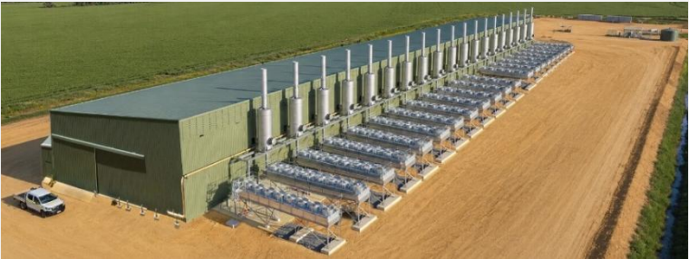
85MW WA power station
