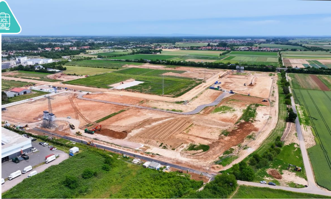
Lionheart lithium extraction site (bottom half of the image) and geothermal power plant site (top right) in Landau.
