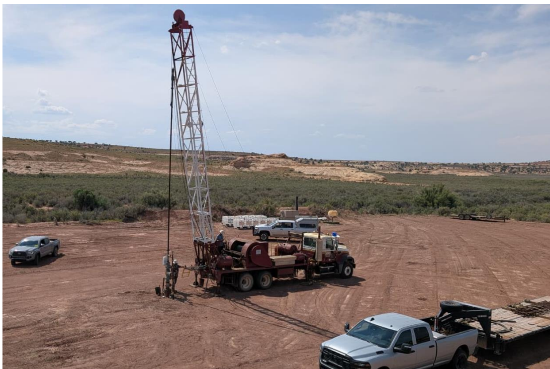
Figure 1: Swabbing unit at the Evelyn Chambers #1 brine extraction well
