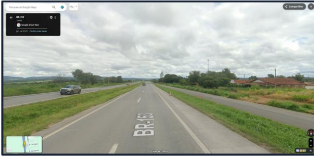
Figure 2: Condition of State Highway BR-153 (Belém–Brasília Highway), the main connection corridor between the region and the state capital, Goiânia. Source: Google Maps – Street View (2025).
