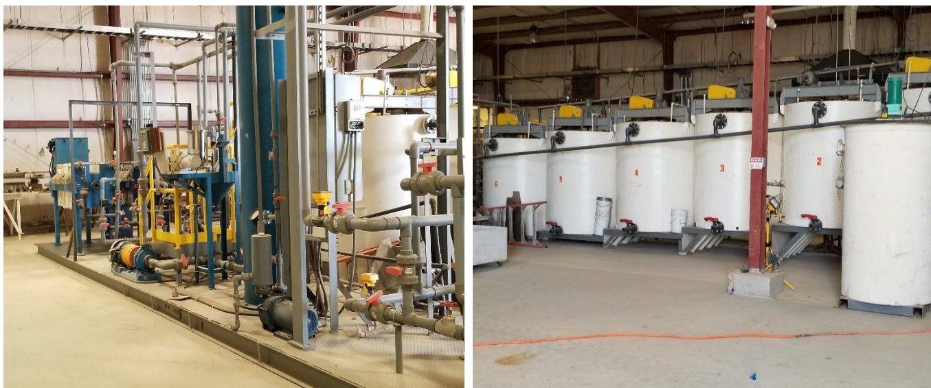
Figure 1 & 2: Infrastructure at the Del Sol facility
