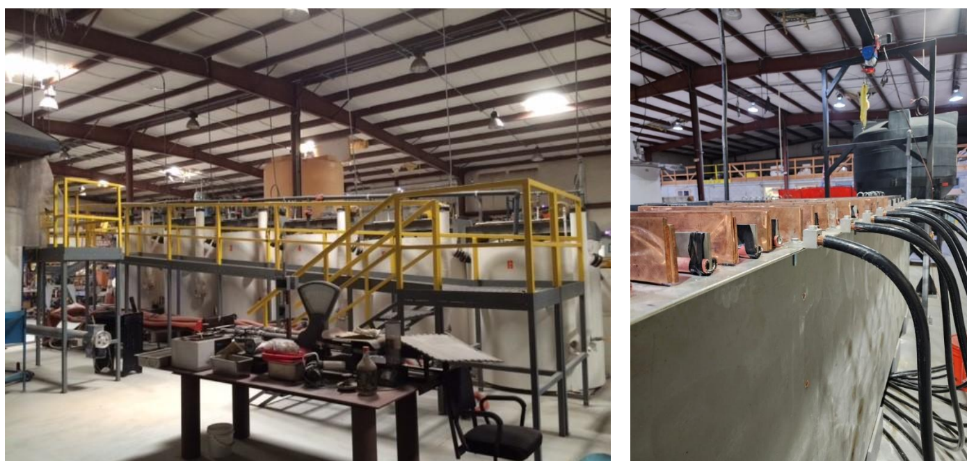
Figure 3 & 4: Infrastructure at the Del Sol facility
