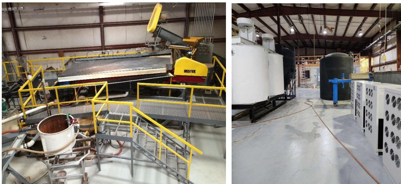
Figure 5 & 6: Infrastructure at the Del Sol facility
