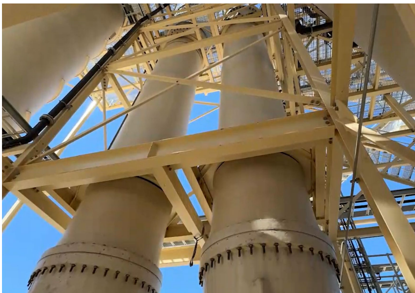
The CLEAN-IX® U-Column plant is in commercial operation at Heathgate.
