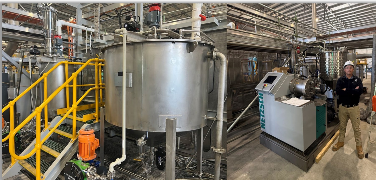
Installed HPA nano-mill and supporting equipment
